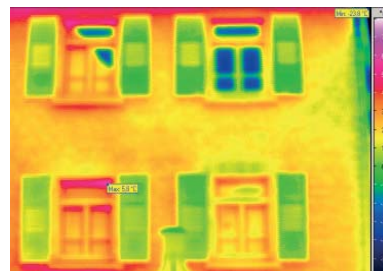
1b: Thermographic image
