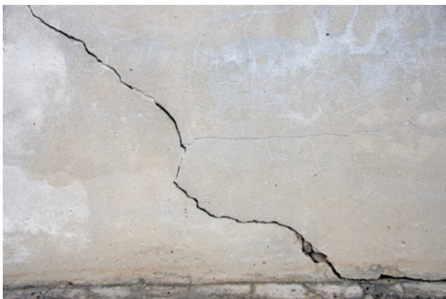
Cracks in the substrate
