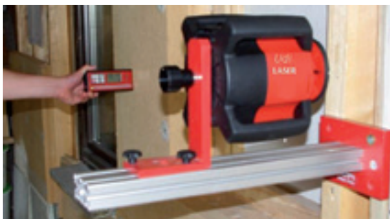
The insulation board can be brought into plumb using a spirit level or laser
