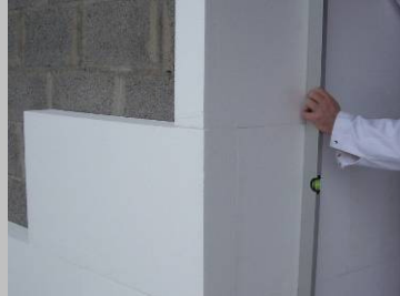
Fig. 9 Check that the boards are plumb and in line. Do not bang the boards.
