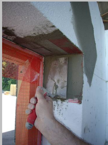
Fig 3 Apply additional reinforcement mesh around internal corner of head and reveal in a tight coat of bonding mortar.
