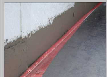
Step 14 Apply a full layer of base coat mortar behind the mesh strip.
