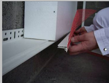
Step 9 Starting at one end, line up the drip bead with the lip of the base profile and push in tight up to the insulation board
