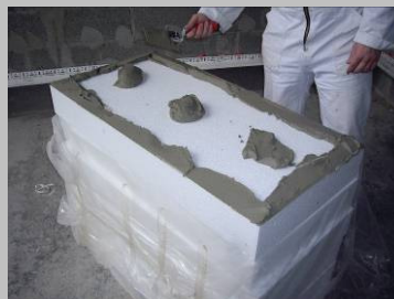
Fig. 3 Apply 3 equally spaced adhesive mortar dabs through the centre line of the insulation board and a strip around the edge.
