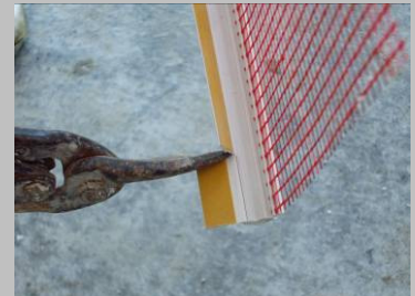
Step 4 Cut and fit the seal bead for the head of the window frame.
