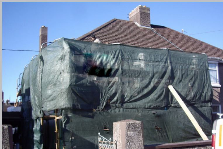
Step 6 Protect the newly rendered façade until set and dry, this will be 2-3 days approx in normal weather conditions.
