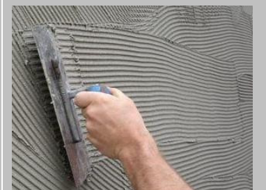
Step 4 Comb through the mortar with a notched trowel to set a uniform depth of thickness.
