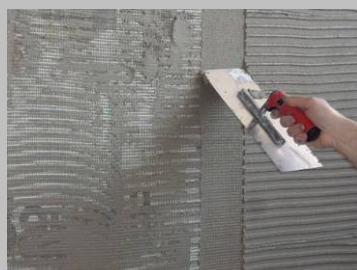
Step 7 Press the edge of the mesh sheet a little deeper into the mortar with the tip of the trowel.
