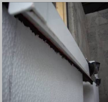
Step 5 Band is also required under the sill, and must sit flush with the board surface.
