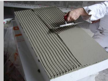
Fig. 5 Apply a full coat of adhesive mortar onto the insulation board surface and comb through with a stainless steel notched trowel.
