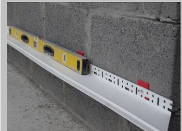
Step 4 Check for level with a long spirit level and continue fixing.
