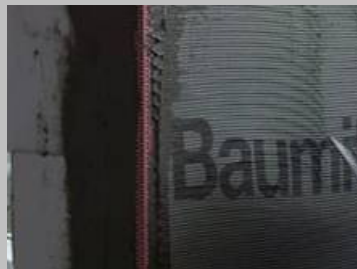
Step 5 Starting 30mm in from the corner edge of the angle bead, lay the mesh sheet lightly onto the mortar.
