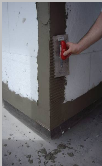
Step 5 Apply a full bed of mortar approx 150mm wide and comb through with a notched trowel to set the depth for the angle bead.
