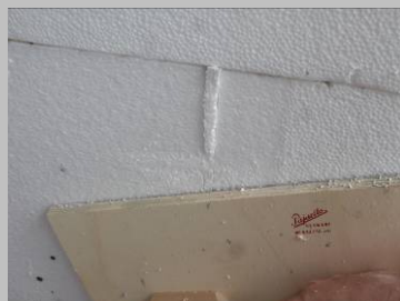
Fig. 15 Rasp back the surface of the insulation boards, removing all undulations leaving a smooth flat surface.
