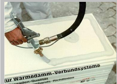
Fig. 4 A direct mix and application from a mortar pump with a pistol attachment speeds up the application of the adhesive mortar to the board.
