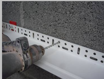
Step 1 Starting at one end; drill a bore hole into the substrate through the perforated upstand on the L-section.
