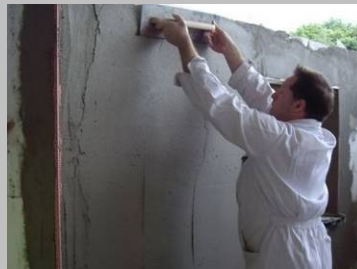
Step 3 Spray or hand apply the bonding mortar over the surface and smooth out with a trowel or plastering rule.
