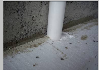
Fig. 6 Buried service pipe
