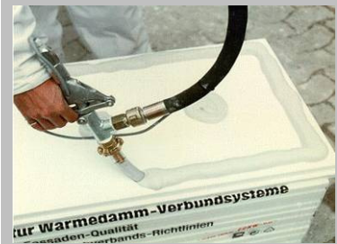
Fig. 4 A direct mix and application from a mortar pump with a pistol attachment speeds up the application of the adhesive mortar to the board.
